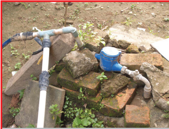
Customers aware of poor service caused by water losses will report defective connections.
